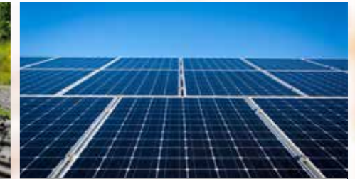
SOLAR POWER PLANTS
